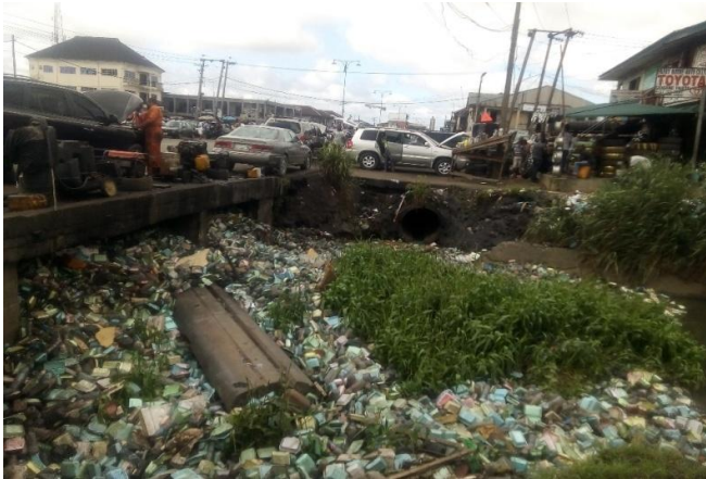
Fig. 1. Blockage of drainage channel with plastics and other materials to stop free flow of water along the Ntanwogba creek due to anthropogenic activities
